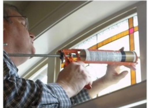
Sealing around windows and doors will help increase comfort in your places of worship.
